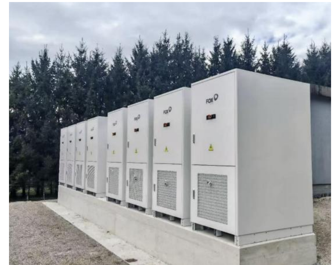
Cabines 115 kW – 230 kWh
