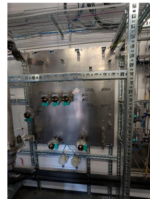
Gas distribution panel
