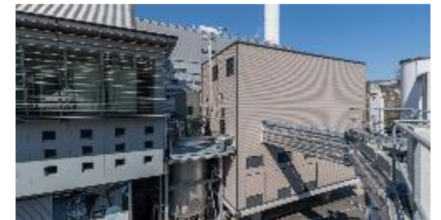
Dietikon/CH, 2.5 MW el PtG (Power-to-Gas) plant, EPC, in operation
