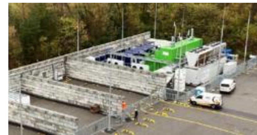
Buchs/CH, 2.8 MW el PtH (Power-to-H 2 ) plant, BOT, in commissioning
