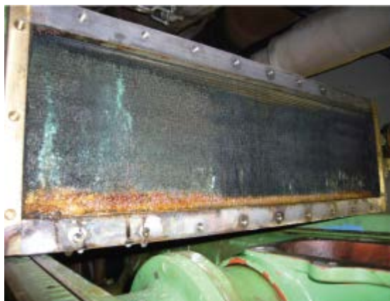
Figure 5: Corrosion de l'intercooler
